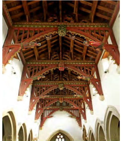
The 'twelve apostles' roof, St John's church, Bere Regis, looking east. (Tony Bates).
